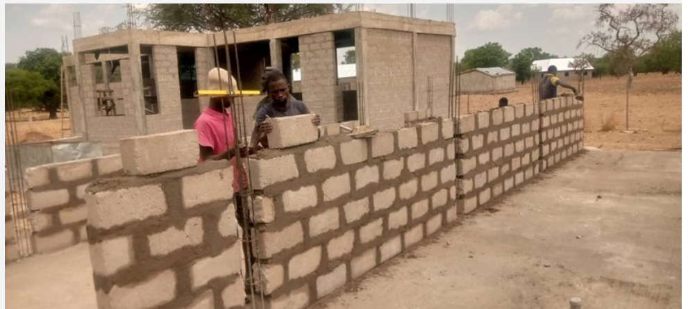
The Food processing building in the background, and the start of the Vegetable 'receiving, washing and cutting' building going up.
